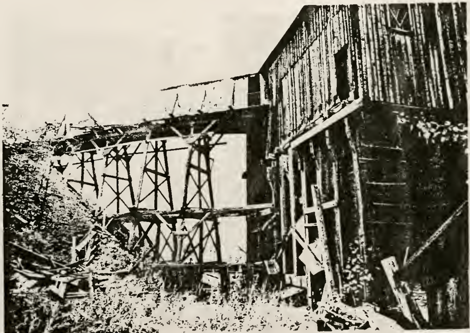
Figure 85. Revenue Mill (structure #34), south view showing east side of new bins and former below-grade hopper area.
